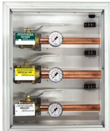
Zone Valve Boxes
