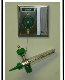
Flowmeter Security Device
